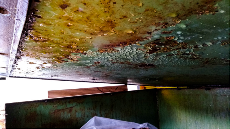
Figure 2 - Inside of the box that showed the highest moisture content. Note the water droplets formed by condensation in the underside of the box lid.
